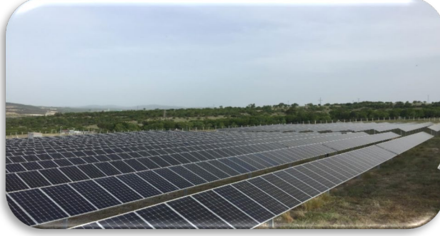
Uşak, Masfen 585 - 1,19 MWp
